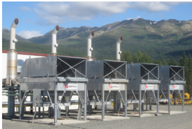
The JBER Landfill Gas Waste-to-Energy Plant was constructed with four generator units designed to run on methane gas produced by the breakdown of wastes buried in the landfill.
