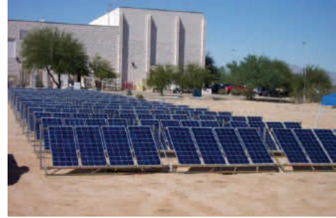
Over the past two years, the AZARNG expanded the use of its most abundant natural energy source: sunlight. The AZARNG's solar projects create over 1 million kilowatts of energy each year.
