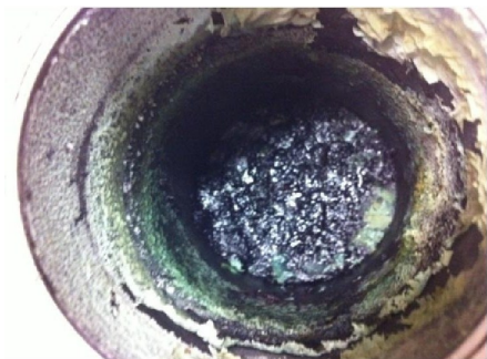
Reactions from counterfeit refrigerants with air conditioning materials can cause equipment, such as laboratory vessels, to corrode.
