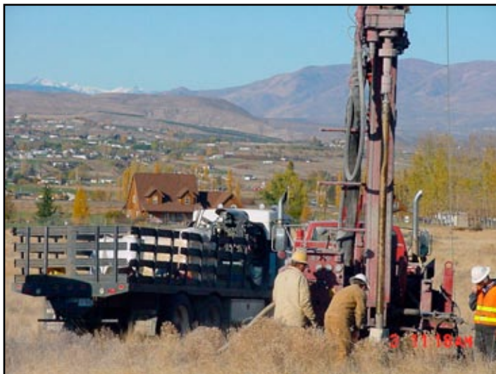
Groundwater monitoring wells are installed as part of an in-house Site Investigation at one of Yakima Training Center's ERP sites.
