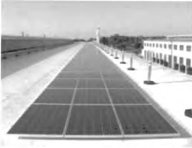
The rooftop of FRCSW Bldg 65, provided a suitable surface and existing windows which made the addition of photovoltaic (PV), daylight harvesting and smart lighting controls cost effective.
