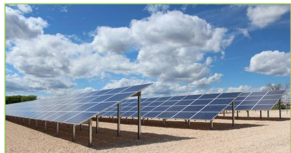
The solar field of 3,000 PV panels will generate 1,000,000 kWh of renewable energy annually.
