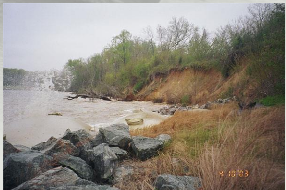
Before: The CAX Site 1 shoreline prior to start of the removal action. Note the steep elevation from the top of the landfill to the shoreline.
