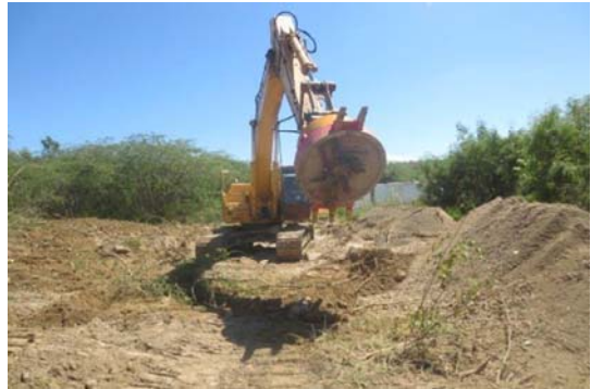
Magnetic attachment on excavator removing bombs from the roadbed. In areas where it is too dangerous or costly to remove munitions by traditional methods, remotely operated equipment has significantly reduced explosive hazards to workers and cut costs by more than half.
