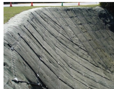
The failed slope near Classroom 1 at the JWTC was effectively stabilized with the use of soil nailing and vegetation matting.
