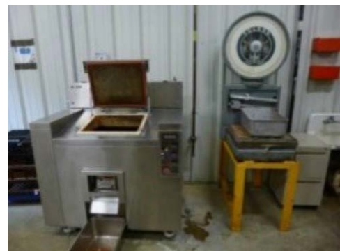
A food dehydrator at Camp Henry DFAC was installed to reduce the volume of food waste generated.
