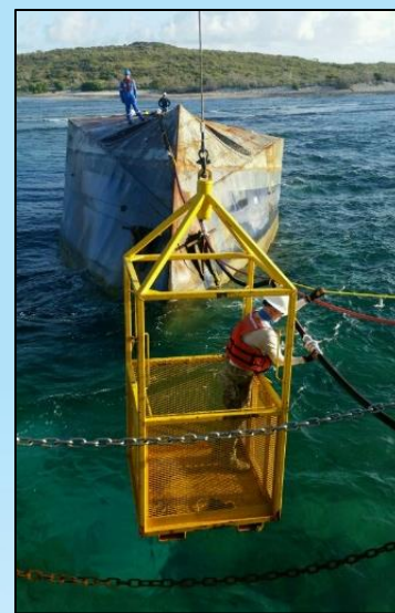
Figure 4. The Navy and its munitions-response contractor provided munitions avoidance and other logistical support to the US Coast Guard during fuel removal from the capsized Ferrel to avoid a release to the surrounding marine environment.
