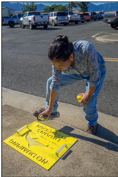
Ms. Xu-Sadri, GS-11 Environmental Engineer, applies a stencil to the side walk just above a storm drain inlet in the industrial and maintenance area of Marine Corps Base Hawai'i that reads, "No Dumping...Drains to Ocean."
