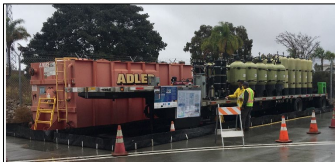
MCAS Miramar employs a trailer-mounted treatment system to remove PFAS from AFFF-contaminated wastewater to below LHA and RSLs.
