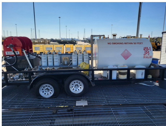
The Fuel Filtration Unit at MCSF-BI, with several off-spec JP-5 totes visible in the background. The fuel filtration unit (FFU) can process most off-spec fuel generated at MCSF-BI. However, contaminated fuel cannot be processed through FFU, and is turned in to the Mayport Base Operating Support contractor for management as waste.
