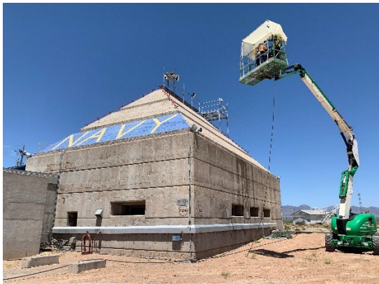
Work being performed at the 1945 Navy Blockhouse including pressure washing, removal of previous caulking, and application of multiple non-invasive products.
