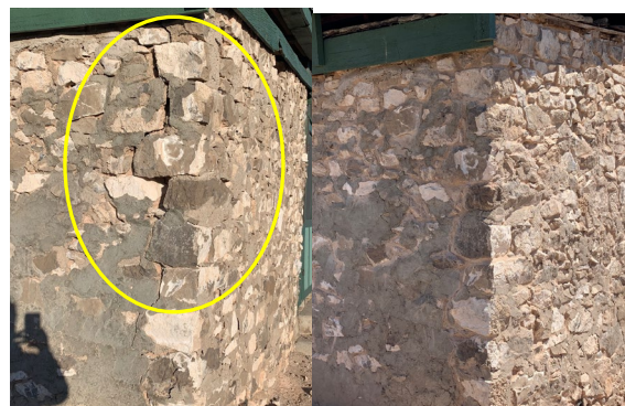
Left illustrating serious masonry failure, right after reconstruction/repair, which included interior bracing and blocking support.
