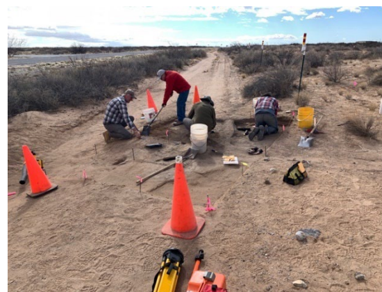
OCA performing testing and damage assessment on WSMR Tank Trail. Siebert stakes protecting site boundaries can be seen on right of trail.
