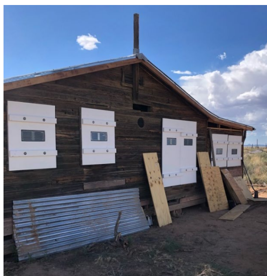
Repaired framed structure to include improved window treatments, siding replacements, and rebuilt/framed/reinforced roof.
