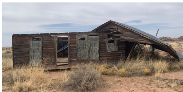
Severely damaged structure from windstorm at Trinity Base Camp NHL.
