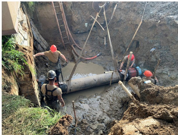
Osan Environmental coordinated closely with the Operations Flight to contain the controlled release of one million gallons of raw sewage that allowed the necessary repair of the sewer main.
