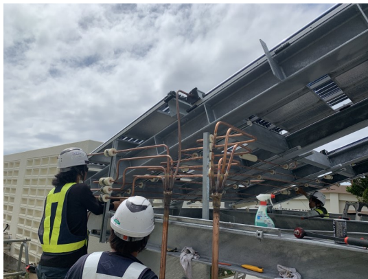
Contractors installing the solar assisted air conditioning unit. This innovative technology is serving as a pilot to evaluate potential application across the rest of the installation.
