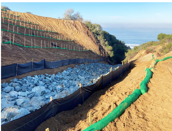
Site restoration in the steep ravine after excavation of solid waste debris and contaminated soil was completed at IR Site 7. Photograph depicts stormwater channel riprap and erosion controls.
