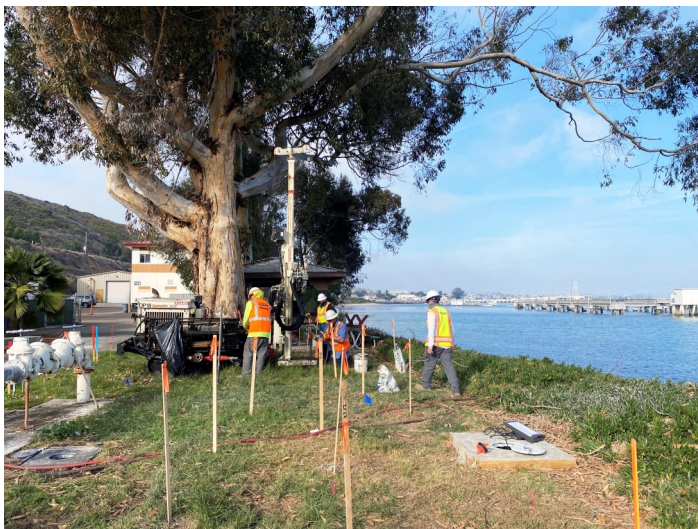
Petrofix injection at UST 105 to implement corrective action for petroleum hydrocarbon release from a former UST.
