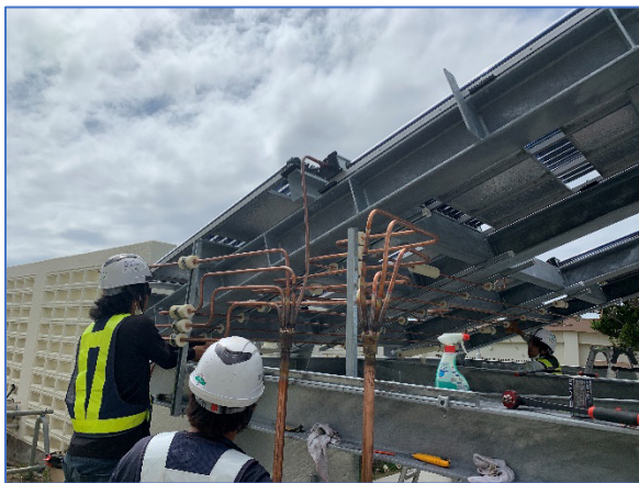
Installation of SolX at Civil Engineering Building Contractors installing the solar assisted air conditioning unit. This innovative technology is serving as a pilot to evaluate potential application across the rest of the installation.
