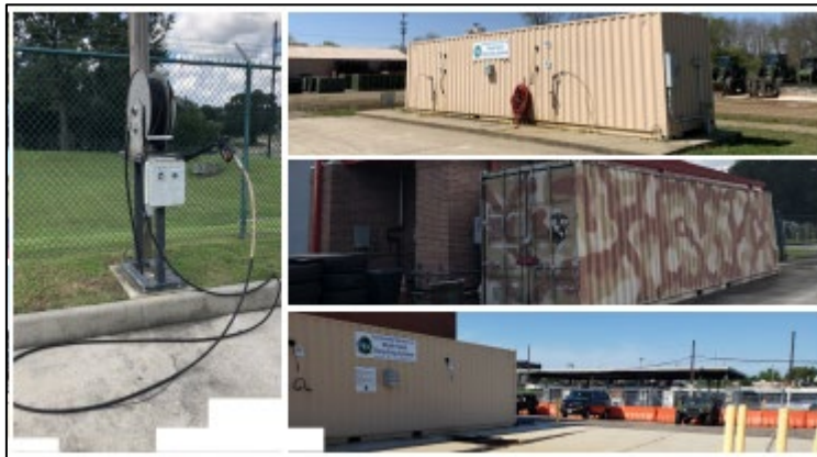
Closed-Looped, recycled water systems
