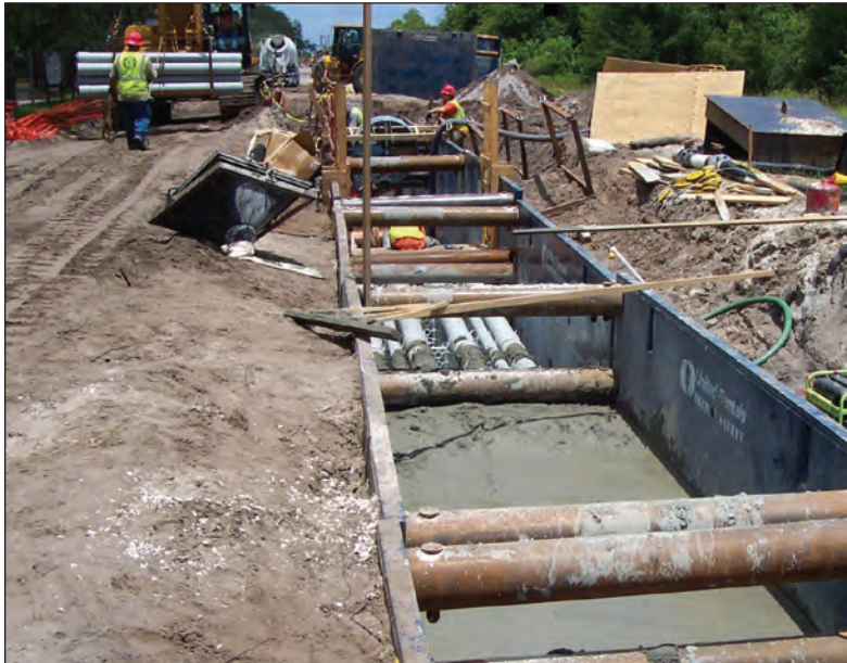
FIGURE 5.6: Buried power lines may be a solution to bird collisions in some instances, but can cost from 3 to 20 times more than overhead lines and have other environmental impacts.
