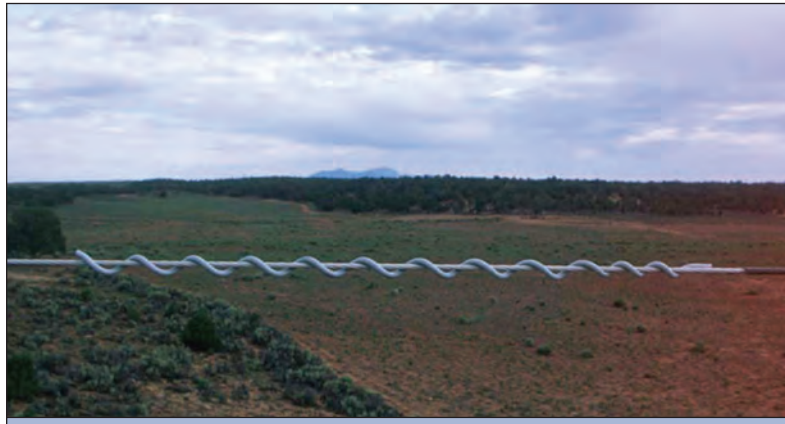
FIGURE 6.10: Spiral vibration dampers act to reduce line vibration, and they also make power lines more visible to birds.
