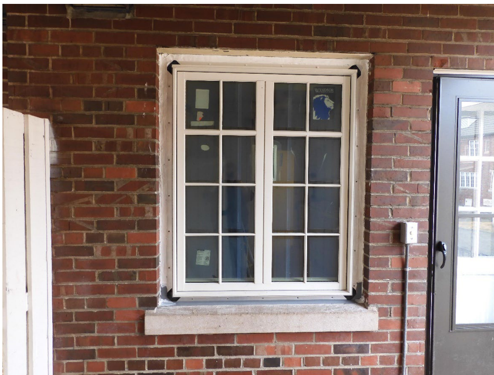
Figure 9: New replacement imitative substitute windows at Joint Base Lewis McChord
