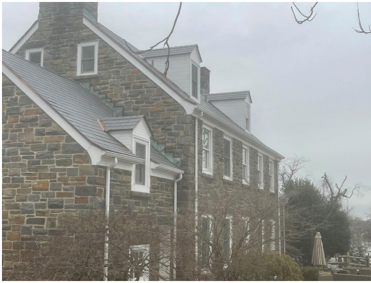
Figure 10: Aberdeen Proving Ground roof replacement using imitative substitute synthetic slate. Cost savings for this one roof replacement resulting from use of synthetic slate vice natural stone slate was over $112,000. Roof replacement required due to significant deterioration of original roofing materials.
