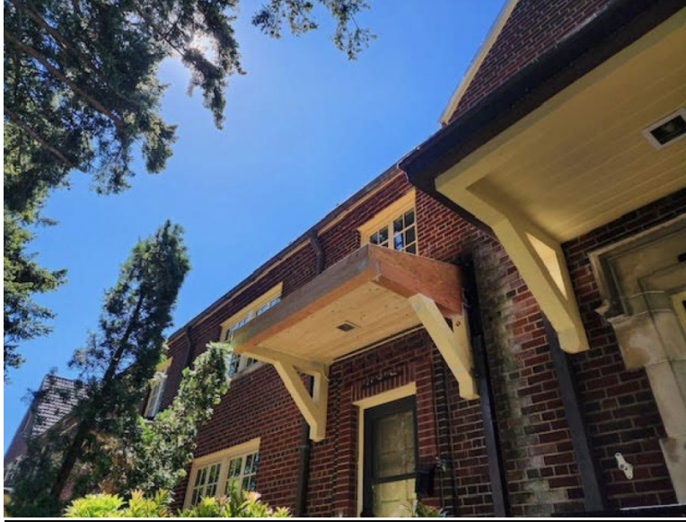
Figure 7: Joint Base Lewis McChord, in-kind replacement of rotting wood on porch overhang, after, 2023
