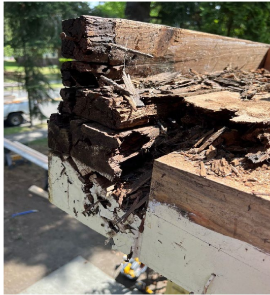
Figure 6: Joint Base Lewis McChord, in-kind replacement of rotting wood on porch overhang, before, 2023
