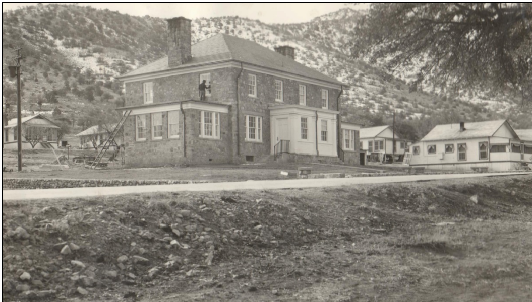
Figure 46. Looking east at the Stone Quarters [21103] during construction, 1939 (NARA College Park, RG 77 entry 394 box 9).
