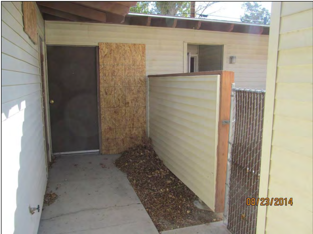
Figure 108: The front entrance to the duplex units. The pony wall to the right separates a graveled courtyard that was used for air drying laundry and accessing the storage structure. The door on the right opens from the kitchen directly into the courtyard. The board by the front door covers a large fixed window that lights the entry area. Photo by S. Simpson, 8/24/2014. (Note: the date on the photo stamp is incorrect.) IMG_0013.jpg.
