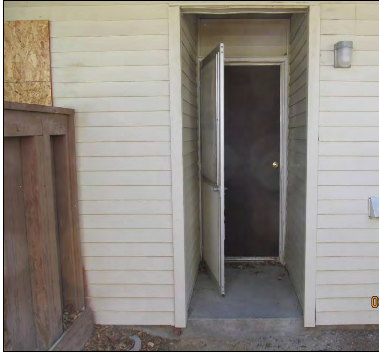
Figure 119: Door exiting from the kitchen into the courtyard. Photo by S. Simpson, 8/24/2014. IMG_0014.jpg.
