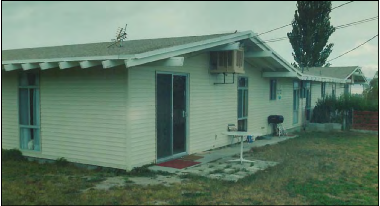
Figure 86: Rear of an unidentified Conelly Duplex after the installation of vinyl siding. The original roof with rafter tails and purlins projecting beyond the drip line is still intact. The roofs were later altered to a composition shingle roof and the rafters and purlins were either shortened, or the roof was extended so they no longer projected beyond the drip line. Photographer and date unknown. (HWAD files, Conelly Duplex Units.)
