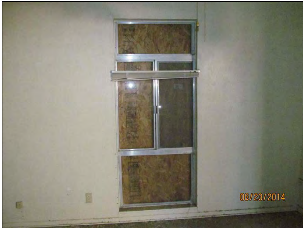
Figure 137: Window in the living room. The upper and lower lites were fixed. The center lites are sliders. The wood baseboard molding appears original throughout the house. Photo by S. Simpson, 8/24/2014 (Note: date stamp on photo is incorrect.) IMG_0028.jpg
