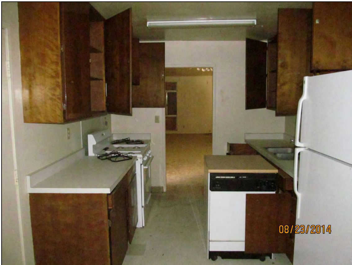
Figure 25: The kitchen, with original wood cabinetry, is accessed from the living room (seen in the background). Photo by S. Simpson, 8/24/2014 (Note: date stamp on photo is incorrect.) IMG_0025.jpg
