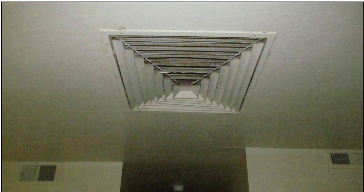
Figure 31: Vent for the evaporative cooler. Photo by S. Simpson, 8/24/2014. IMG_0026.jpg.
