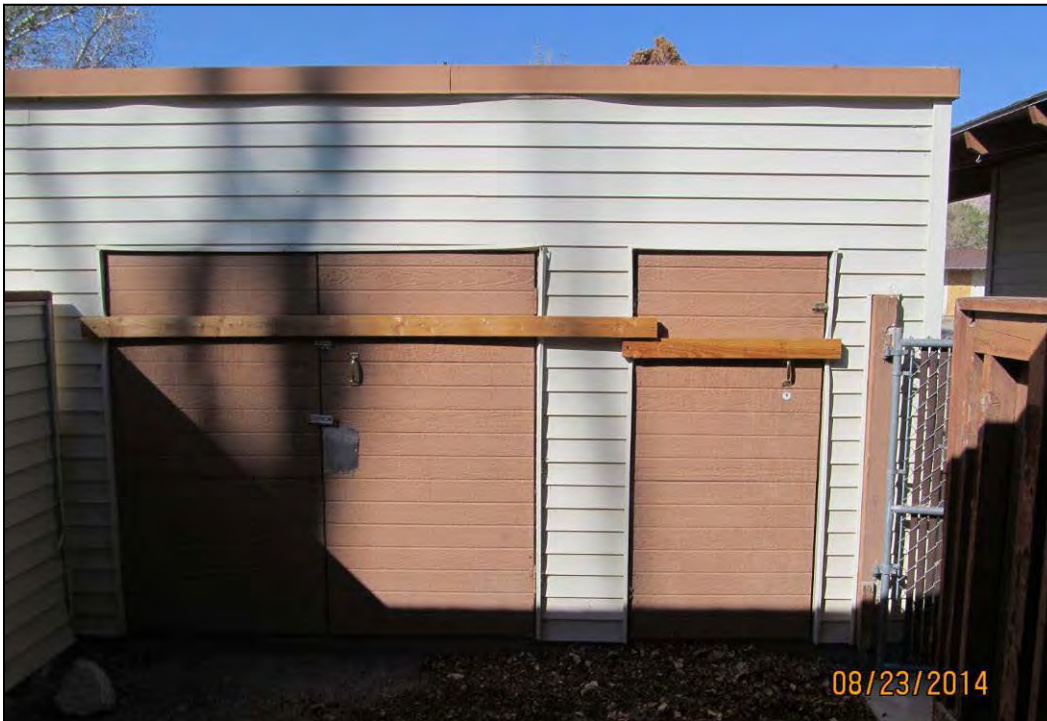
Figure 22: Interior of the courtyard showing the storage building. (Note: date stamp on photo is incorrect.) IMG_0016.jpg
