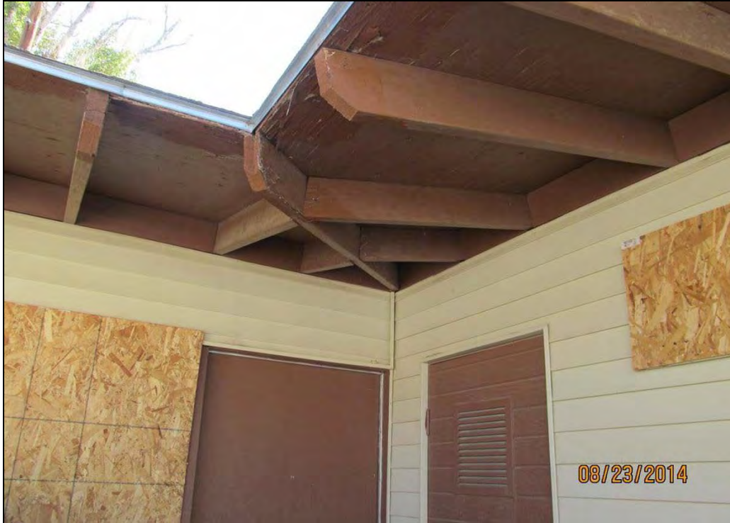
Figure 21: Roofing detail. The original rafters were not clipped, as seen here. Photo by S. Simpson, 8/24/2014 (Note: date stamp on photo is incorrect.) IMG_0055.jpg
