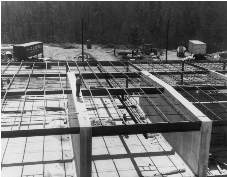
Figure 45. View of construction of Ammunition Maintenance Facility at Fort McClellan, Alabama, June 1975 (NARA SC671011).
