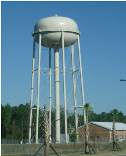
This is a 250,000 gallon storage tank for the Lower Floridan well located in the 2nd Infantry Brigade Combat Team area on Fort Stewart. This is one of several tanks tied to a loop system, meaning the tank can be supplied by any of the wells on Fort Stewart.
