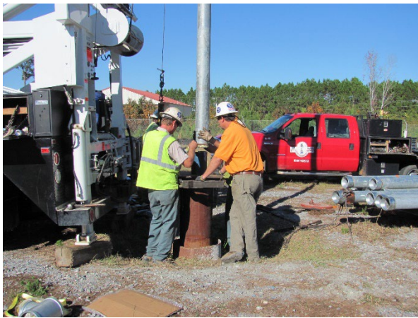
The Lower Floridan Aquifer well being drilled at HAAF. Workers shown here during the installation of a pipe which is attached to the submersible pump. This well was drilled to ~1100 feet.
