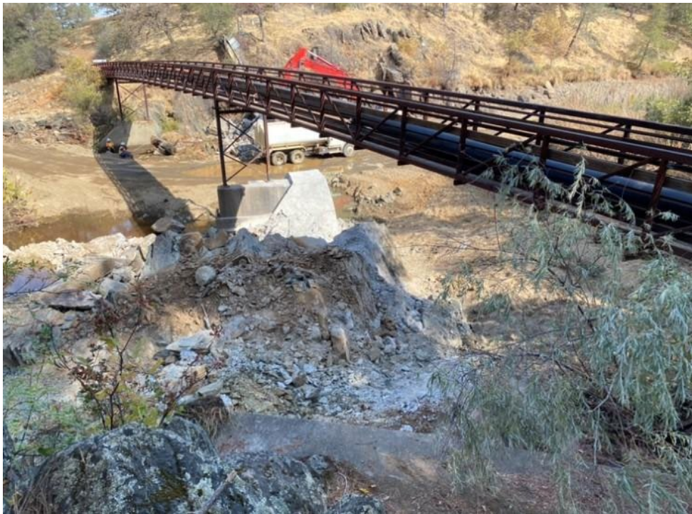
Figure 6-3. Beale Dam demolition at 95% complete at Beale AFB, California in August 2020. (Figure by Kirsten Christopherson, Air Force Civil Engineer Center, Travis Installation Support Section)
