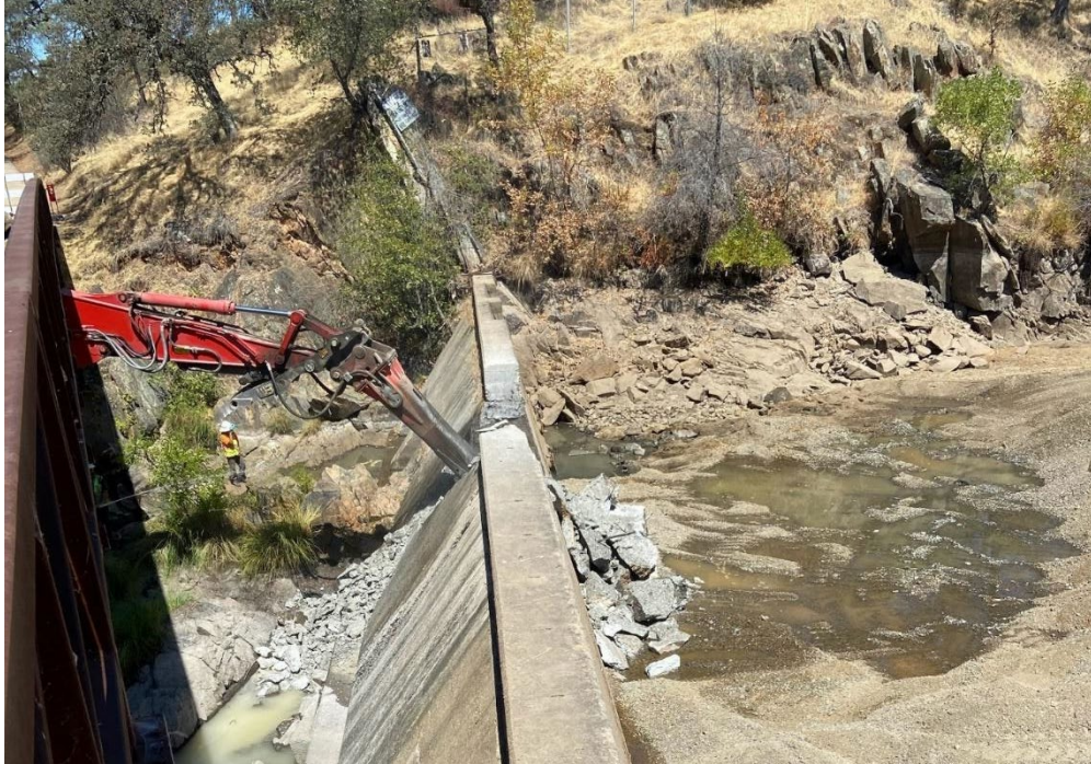
Photo 6-2. First day of Beale dam demolition at Beale AFB, California in July 2020. (Photo by Chadwick McCready, Colorado State University, Center for Environmental Management on Military Lands (CEMML).
