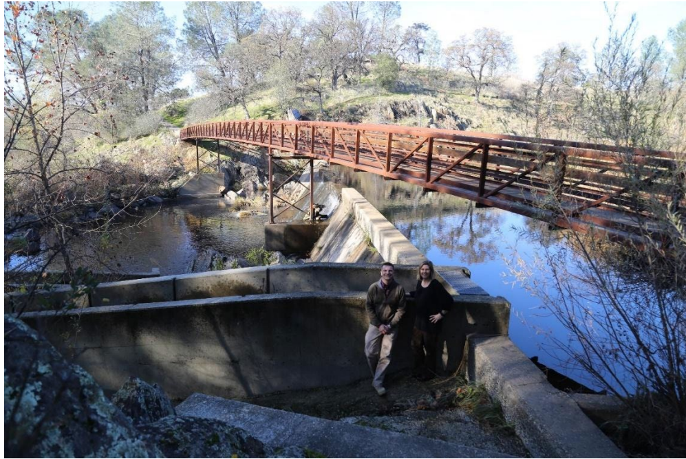
Figure 6-1. Beale Dam, fish ladder, and pedestrian bridge on Beale AFB, California in December 2017 prior to dam removal. Pictured: Jason Gibbons & Kirsten Christopherson, AFCEC, Travis Installation Support Section. (Figure by Kirsten Christopherson).
