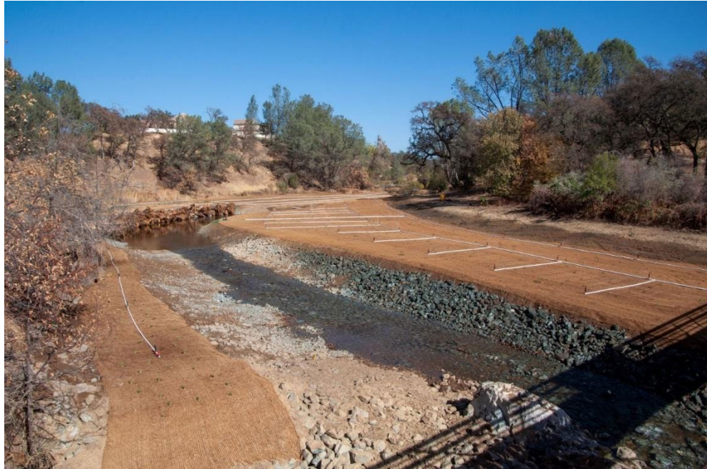
Figure 6-4. Post-construction view looking upstream at the former Beale dam site after removal, but before seasonal rains started at Beale AFB, California in October 2020. The area pictured used to be Beale Lake behind the dam, and is now a rocky, seasonal stream. (Photo by Brandon Honig, U.S. Fish and Wildlife Service, Sacramento, External Affairs Office)
