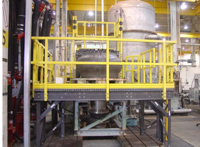
New customized staging promotes access to pumps.
