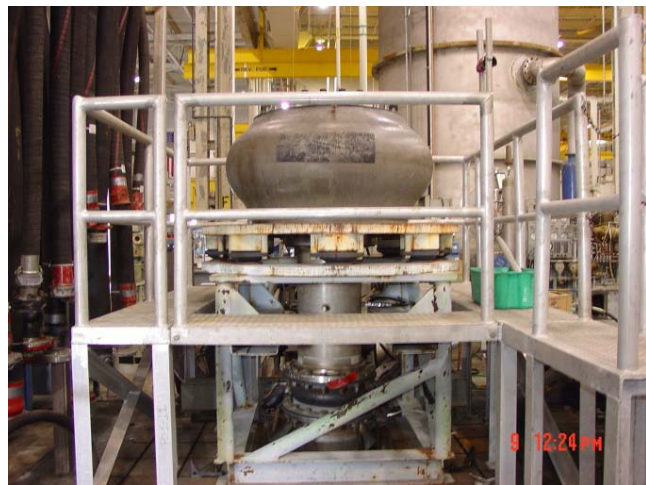
Pump shown in test fixture with temporary staging surrounding it.
