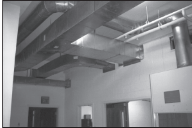
Figure 280. Examples of the environmental and fire protection systems.
