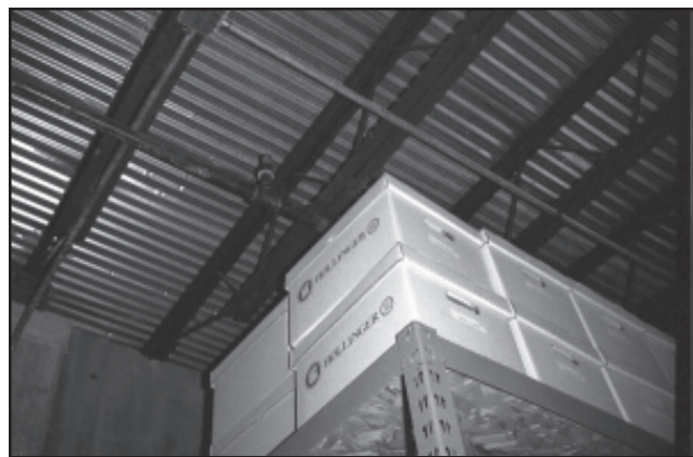
Figure 179. Example of boxes stacked on metal shelves that are located directly beneath a sprinkler head in the collections storage area.
