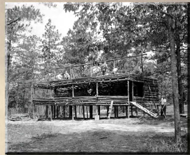
Workers construct a "long house" at Bau Bang training village at Fort Jackson, South Carolina, 1966.
