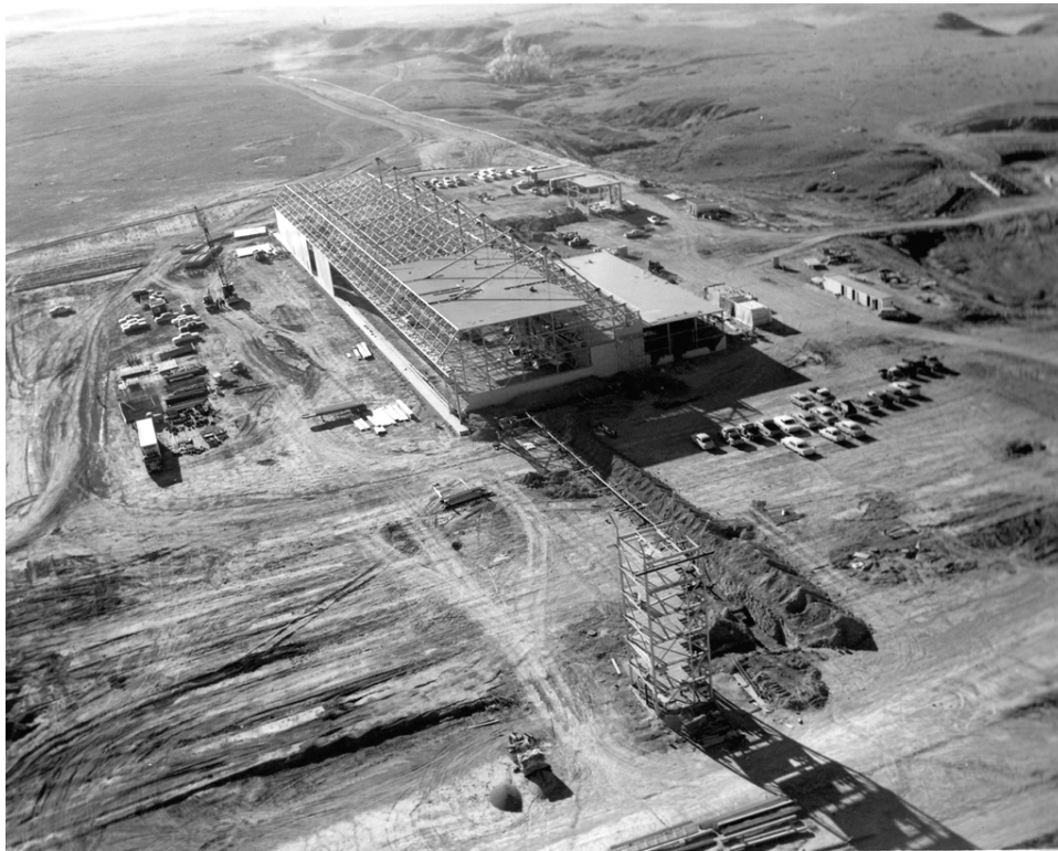
Figure 17. Aerial image showing the construction progress on Butts U.S. Army Airfield facilities, Fort Carson, Colorado, October 1963 (NARA SC 609436).
