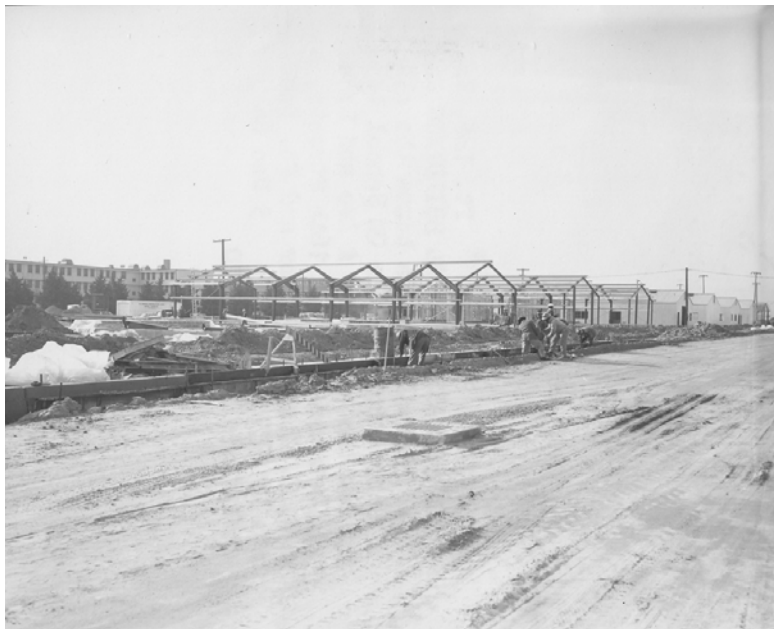
Figure 25. New Quartermaster School buildings under construction at Fort Lee, Virginia, December 1966 (NARA SC635694).
