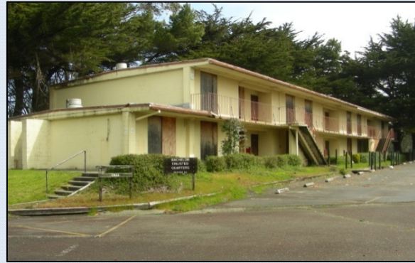
Figure 16: The now demolished 1973 Bachelor Enlisted Quarters (BEQ) at Naval Facilities Centerville Beach near Ferndale, California had a concrete beam frame, concrete slab roof, and concrete masonry unit walls, all of which remained exposed without any attempt at ornamentation (photo: JRP).
