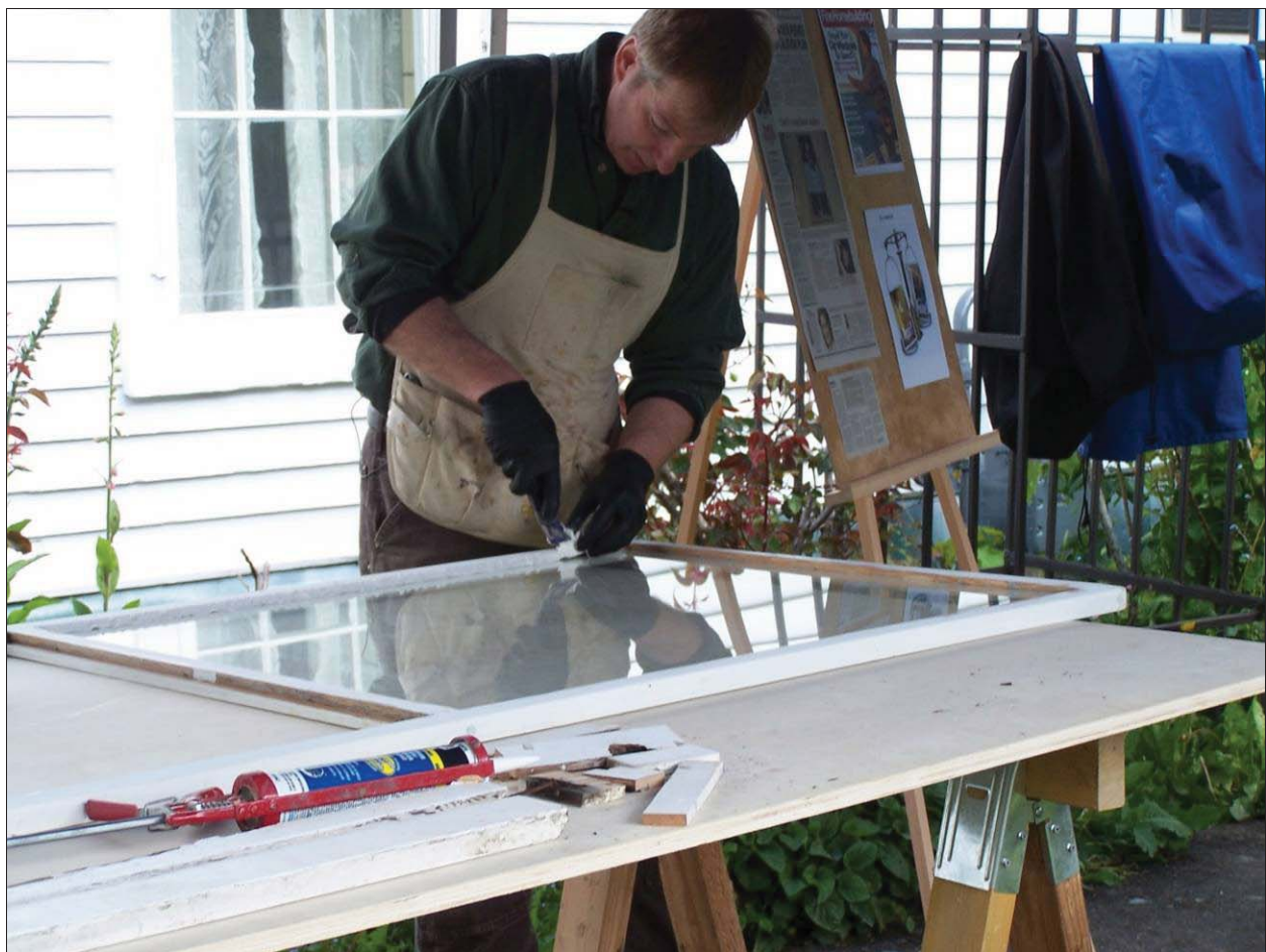
FIGURE 4-26. PHOTO OF THE WOOD WINDOW REPAIR DEMONSTRATION AT BIGELOW HOUSE IN OLYMPIA, WASHINGTON.
