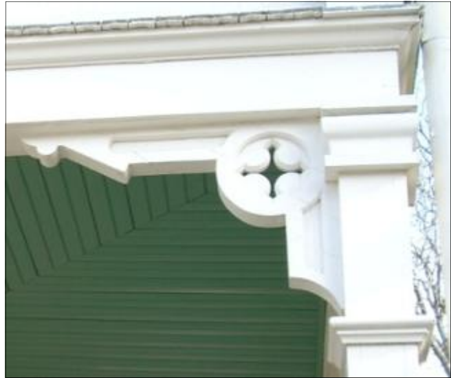
Intricate wood details add character to a historic building. Fort Sam Houston, Texas
