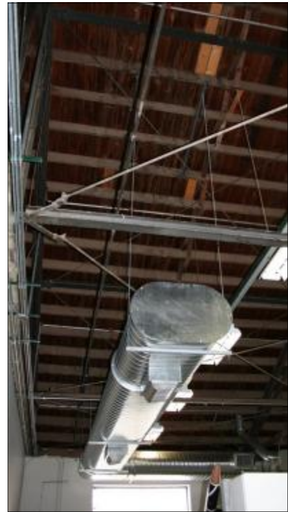
The placement of new HVAC is sensitive to the historic exposed wood structural system.
