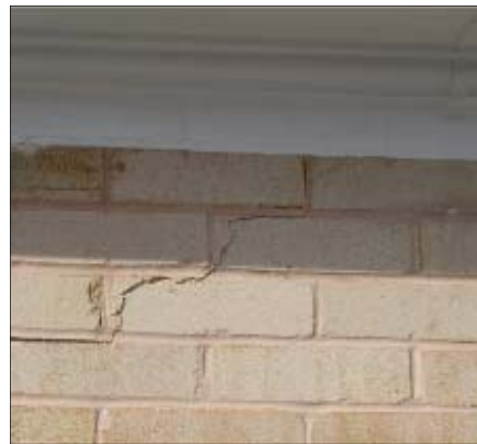
Inspections should closely monitor minor cracks to avoid potential structural problems in the future. Photo courtesy of the Department of the Navy
