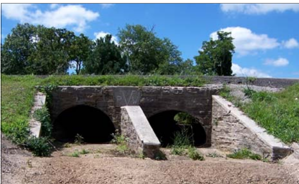
Historic limestone culverts create architectural interest in historic districts. Fort Leonard Wood, Missouri Photo courtesy of ERDC-CERL
