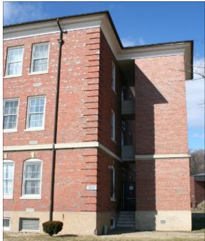
Reversible and compatible addition to this building provides exterior stairs. Marine Corps Base Quantico, Virginia
