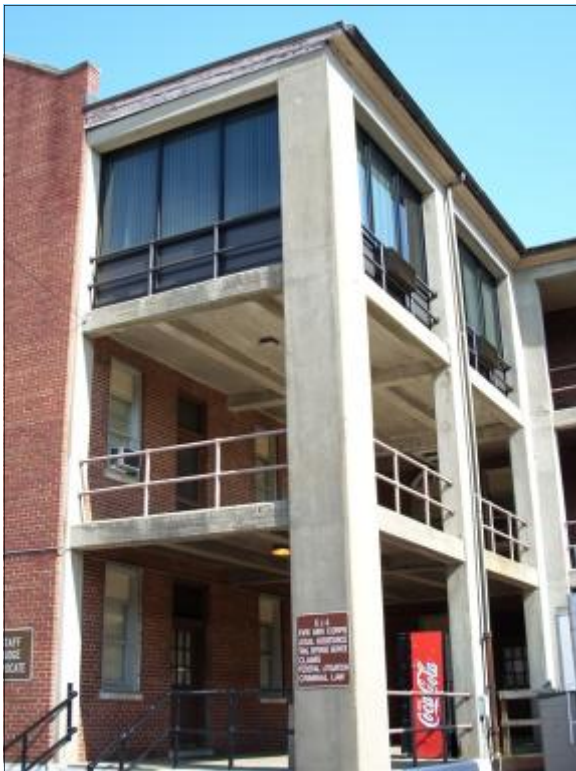
Rear porch was enclosed to provide additional interior office space. The enclosure uses glass placed on the inside of the original porch railings to minimize the impact to the historic building. Fort Bragg, North Carolina
