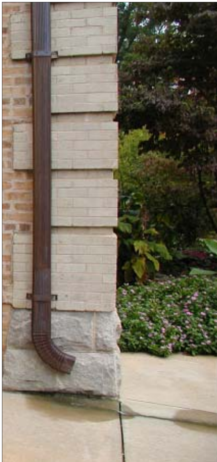
Make sure gutters divert water away from the building. Photo courtesy of the Department of the Navy
