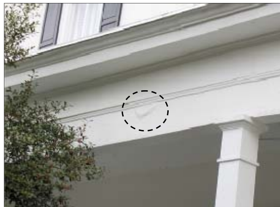
Look closely for potential water intrusions such as leaks in concealed built-in gutters (circled area above). Photo courtesy of the Department of the Navy
