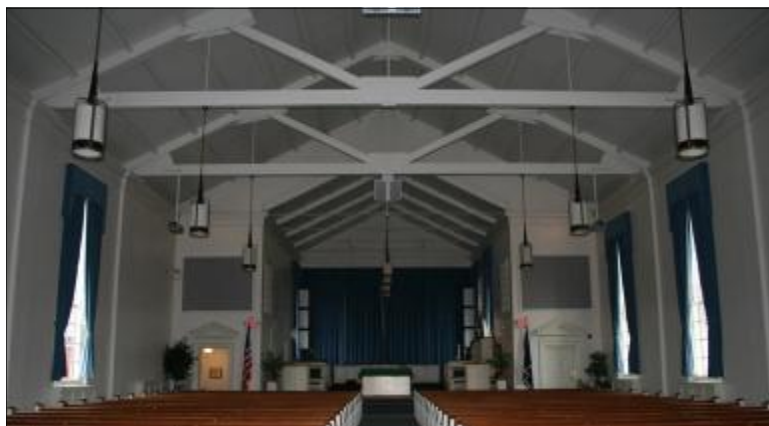
An exposed roof truss enhances the character of a building's interior. Fort Belvoir, Virginia
