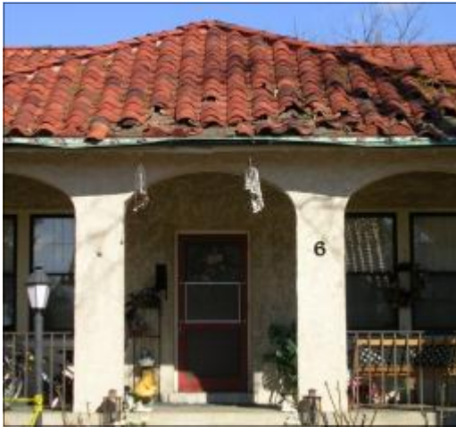
High winds and falling debris can cause roof damage to historic buildings. Fort Bragg, North Carolina Photo courtesy of Fort Bragg CRMP
