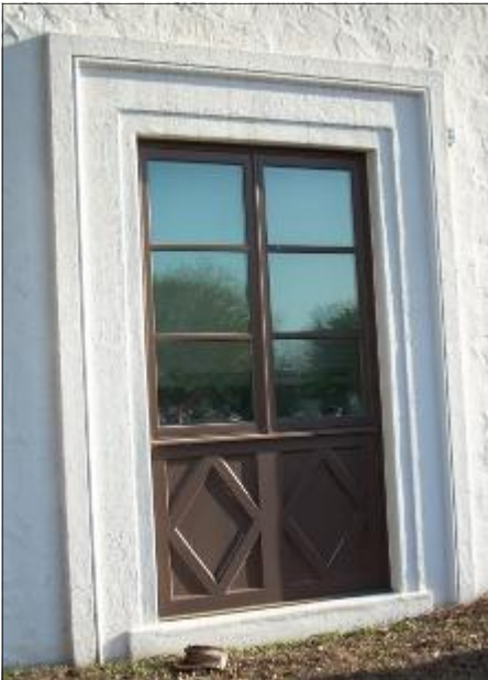
Example of a replacement window that accurately matches the original. Randolph Air Force Base, Texas
