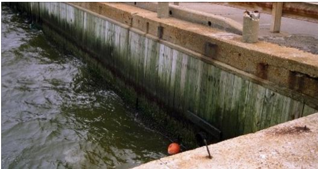
Bulkheads can be important waterfront features and should be protected and preserved. Norfolk Naval Shipyard, Virginia, Photo courtesy of the Department of the Navy
