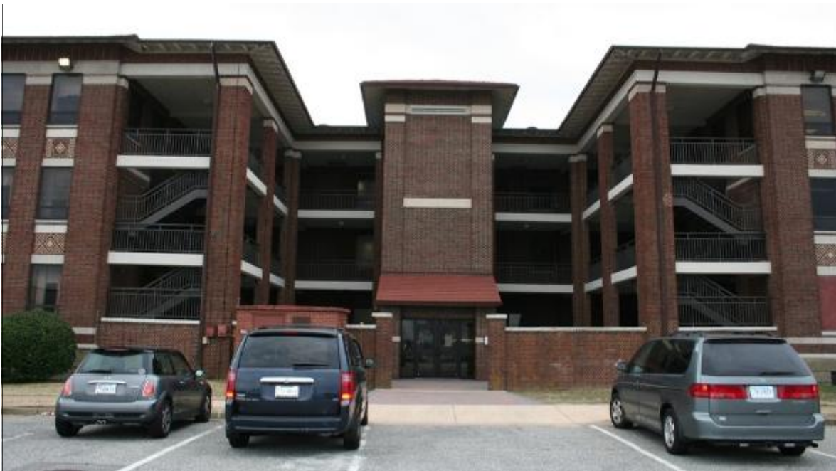
Exterior elevator addition (center) is compatible with the character of the building. Langley Air Force Base, Virginia
