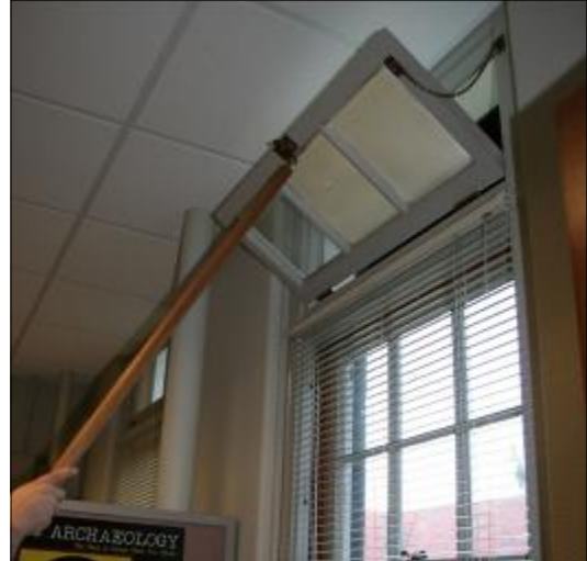
Operating interior transoms can help increase a building's energy efficiency. Fort Lewis, Washington
