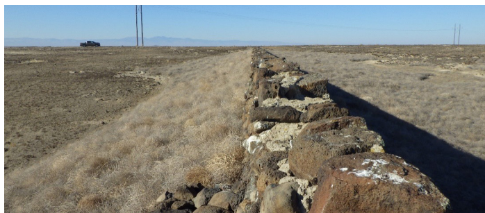
Buildup of hazardous fuels around a historic dam.
