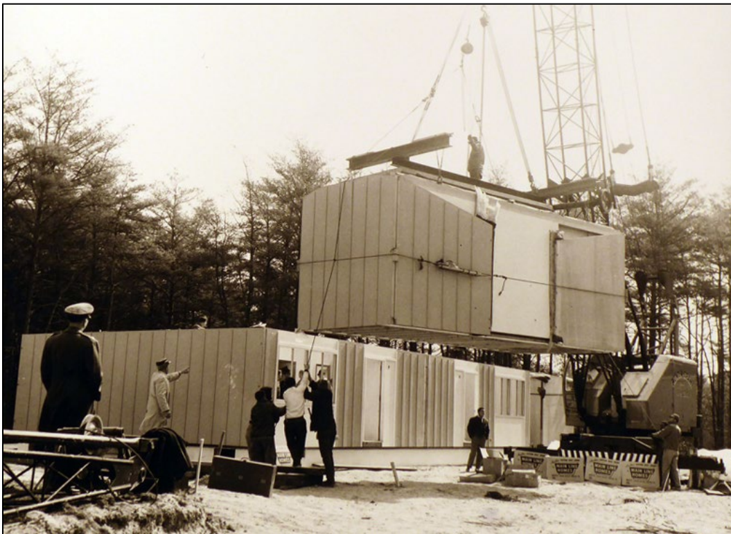
Figure 157. Once the ground floor is complete, the second story is lifted into place in one piece, Andrews AFB, Maryland, 1964 (NARA College Park, RG342-B).
