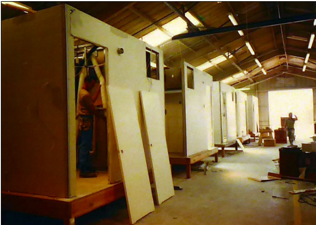
Figure 160. Utility cores being assembled by a line of electricians, plumbers and carpenters, George AFB, California, 1971 (NARA College Park, RG342-B).
