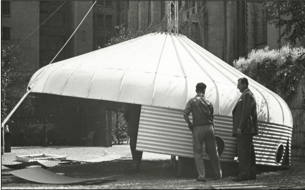
Figure 24. Construction crew beginning to attach horizontally corrugated steel sheet side panels, after raising the conical roof through the circular opening at the top with pulleys (The Museum of Modern Art Archives, New York. IN151.7).
