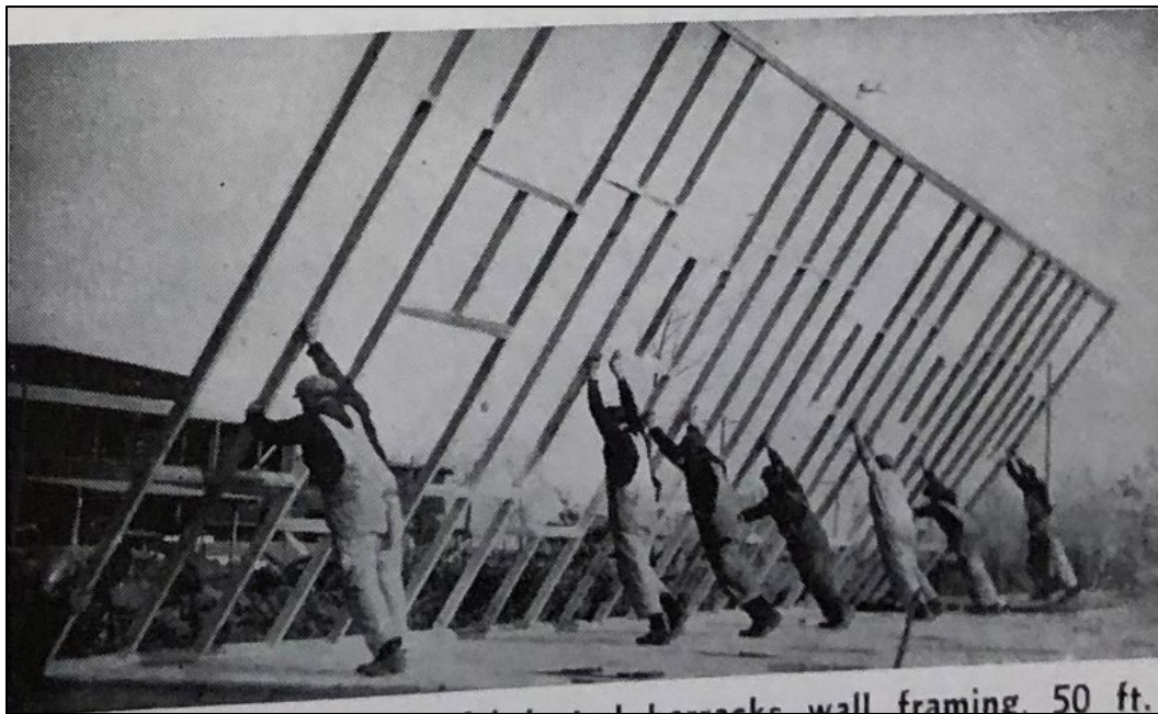
Figure 55. "Complete section of prefabricated barracks wall framing, 50 ft. long and two stories high, being raised into position in from 20 to 30 seconds" ("Prefabricated Naval Hospitals and Housing." Prefabricated Homes 1-5 (Oct. 1944): 14-15 & 21, 15).
