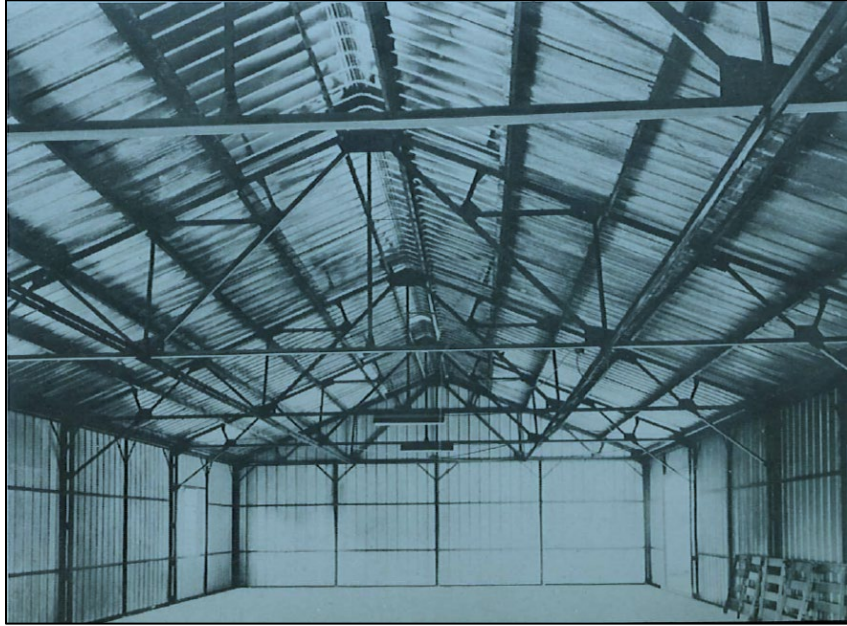
Figure 79. An internal view of the Mesker Prefabricated metal building, providing clear view of Mesker's prefabricated trusses as well as the corner braces along the top of each factory assembled side wall panel (Geo. L. Mesker Steel Corporation, "For economy...for endurance. Mesker Prefabricated Sectional Type Steel Buildings," Evansville, IN: Geo. L. Mesker Steel Corporation, 1959, 4).
