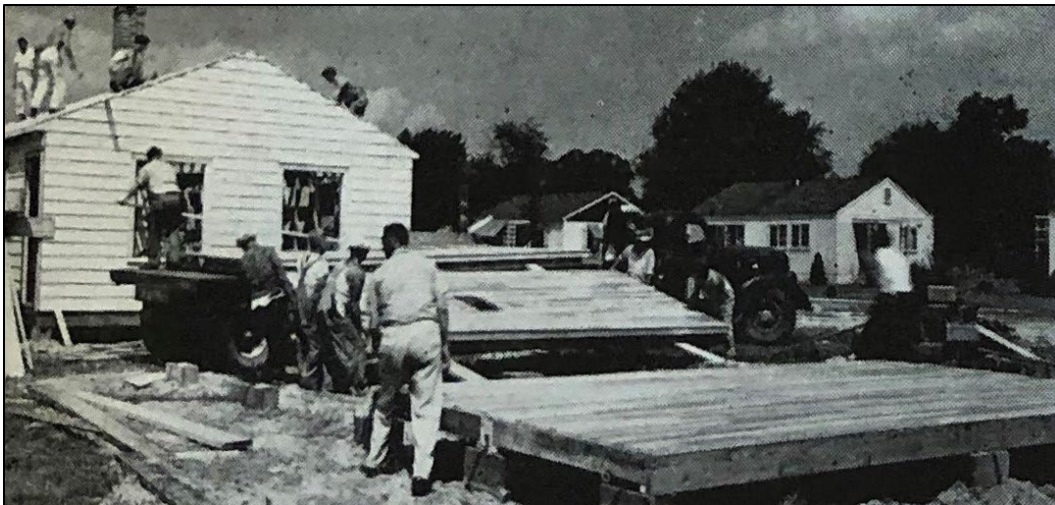
Figure 53. The floor of one of Johnson's prefabricated, demountable "standardized war housing units" is being loaded off the truck and directly into place on the block foundation, showing the level of efficiency sought in on-site construction (John A. Johnson Contracting Corporation, "War speed is typical Johnson Speed!" Prefabricated Homes 1-5 (Feb. 1944), n.p.).
