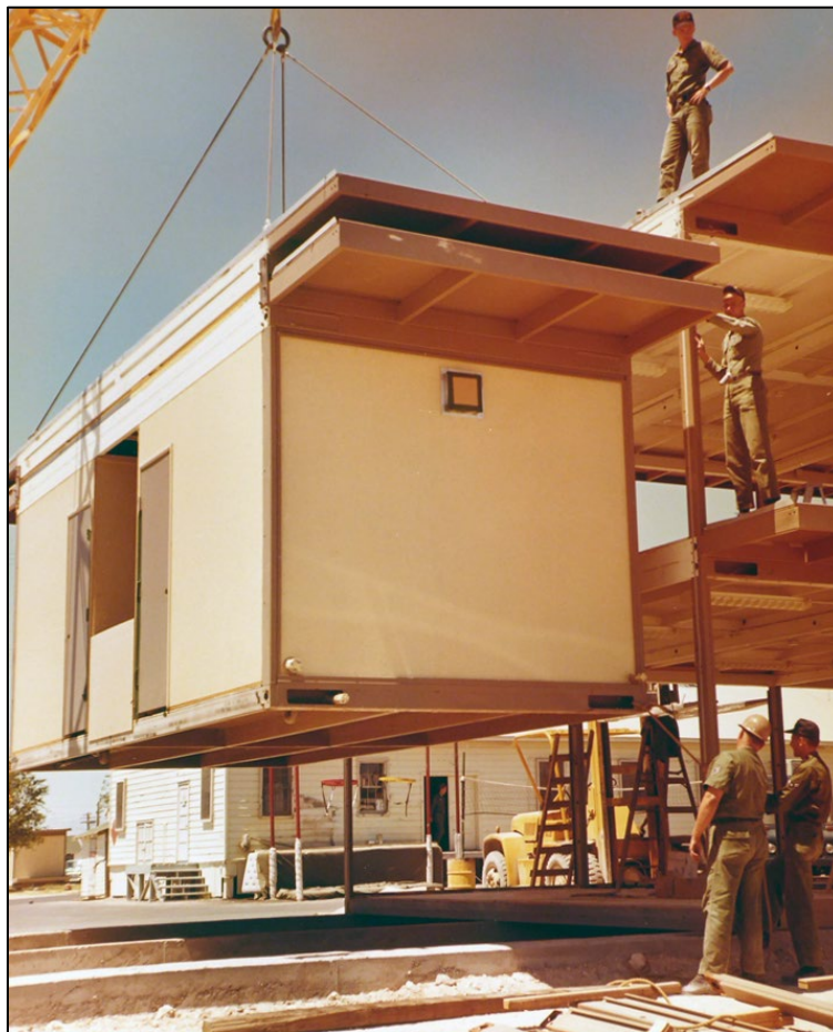
Figure 165. A latrine module being hoisted into place, Nellis AFB, Nevada, 1968 (NARA College Park, RG342-B).
