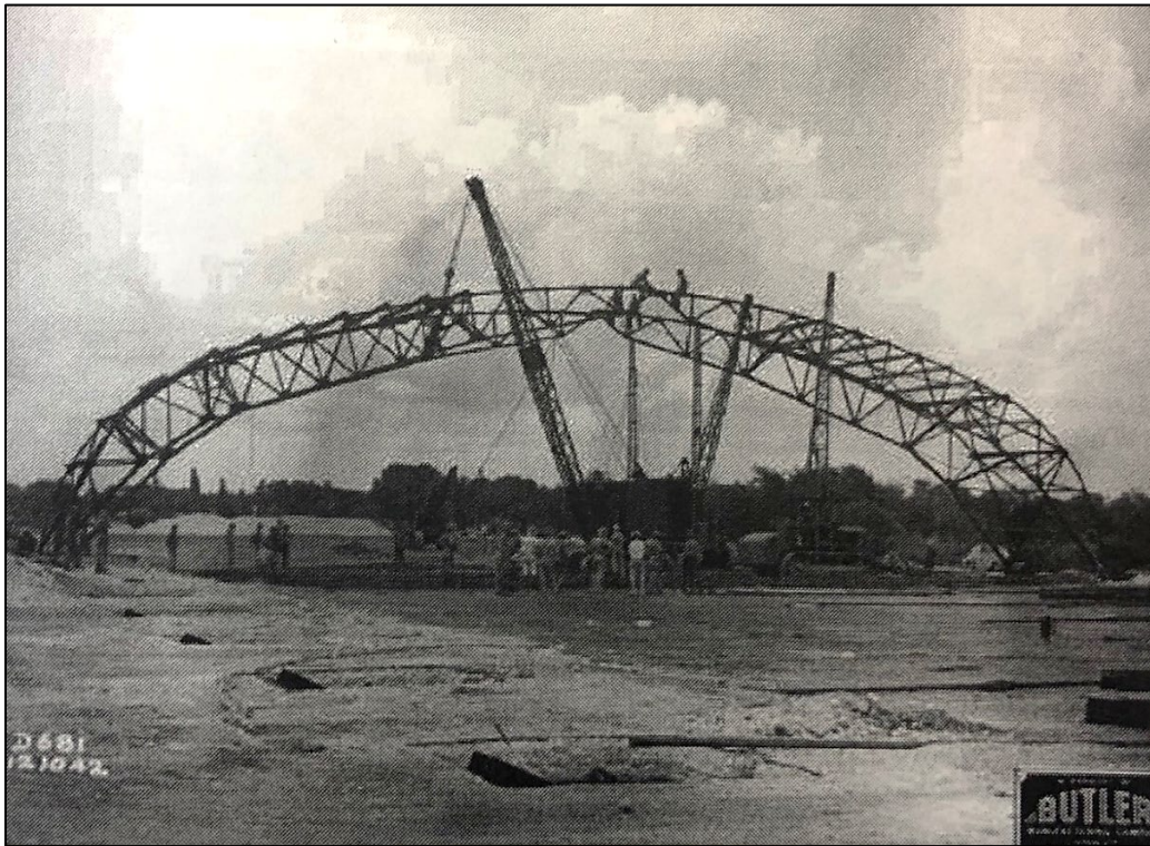
Figure 28. A Butler Manufacturing canvas covered hangar under construction, 1942 (Courtesy of Butler Manufacturing Company Archives).
