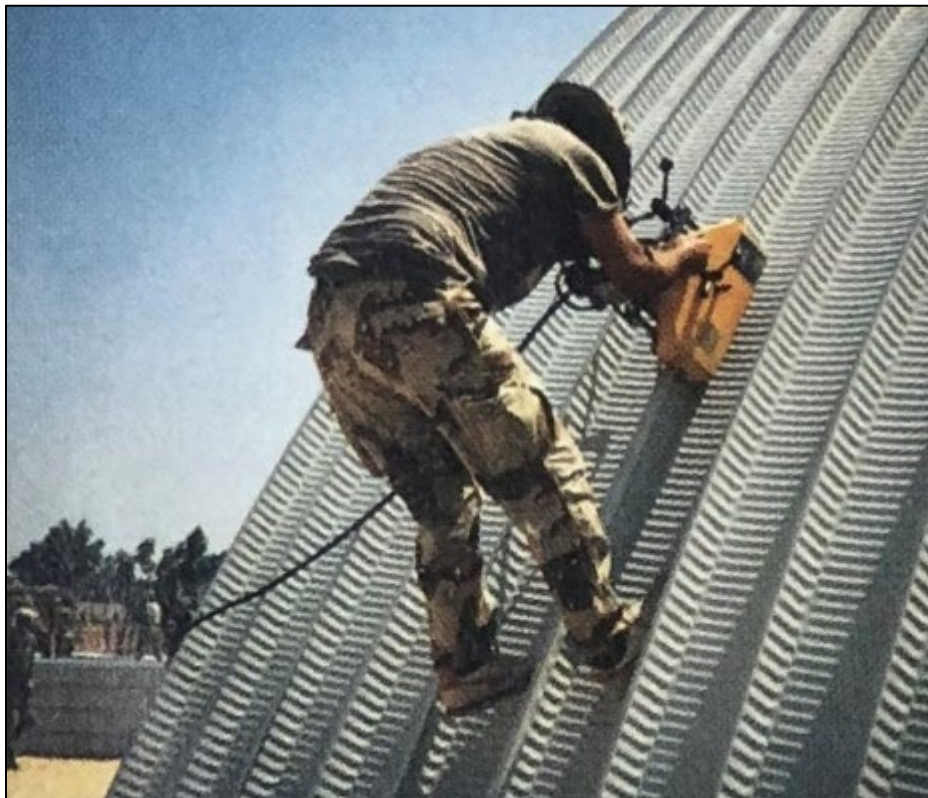
Figure 194. The seam of an ABM structure is being crimped by the automatic seaming machine as it works its way up the side of the structure, 1990 (Forrest T. Gay, "Steel Buildings - On the Double," The Military Engineer 82, no. 535 (May-June 1990): 53-54).
