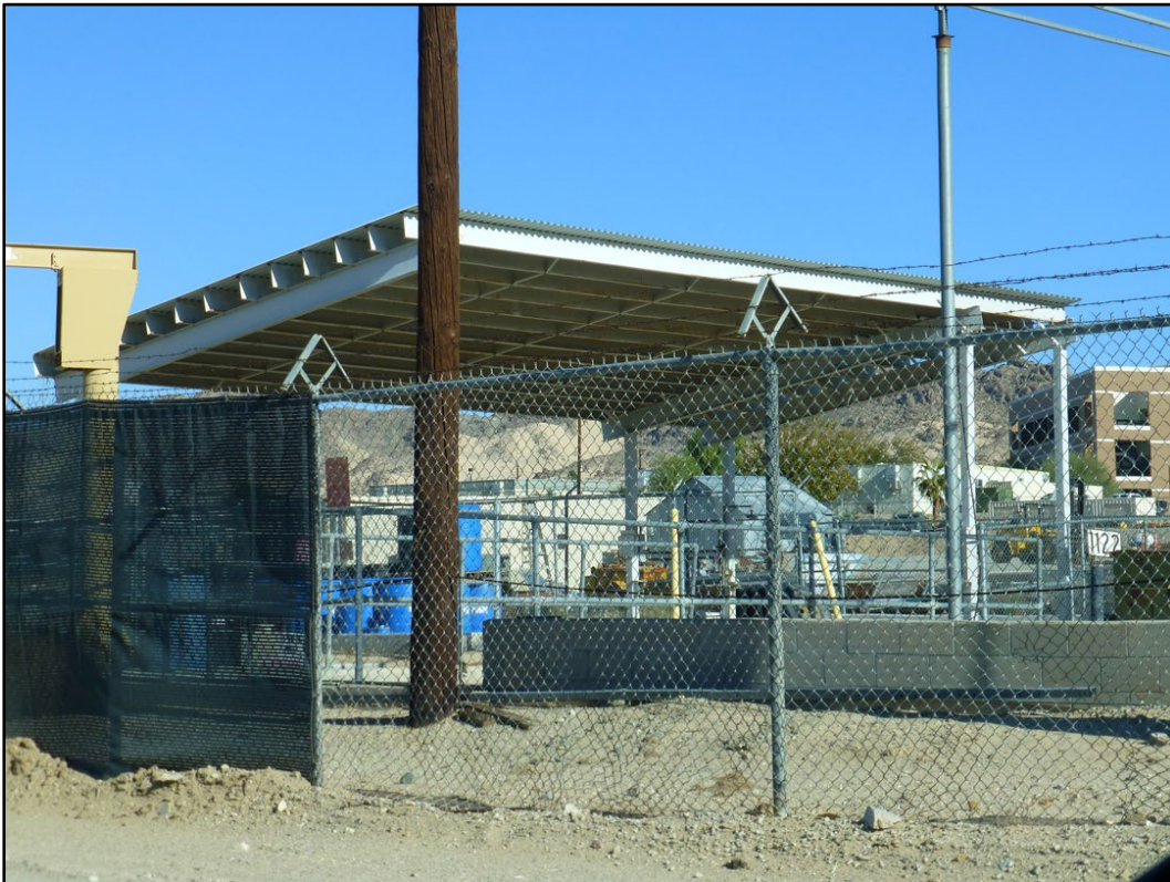
Figure 316. No Number at MCAGCC Twentynine Palms (ERDC-CERL 2016).
