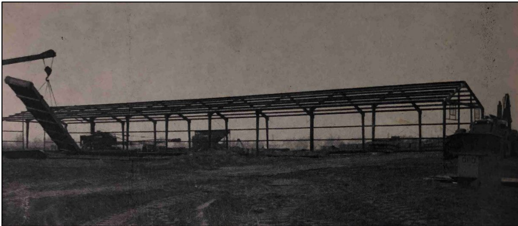
Figure 142. A Butler prefabricated warehouse awaiting siding and roofing at Da Nang, Vietnam (H.N. Wallin, "Military Construction in Vietnam: The Construction Agent," Military Engineer 58, no. 385 (Sept.–Oct. 1966): 317–319, 318).
