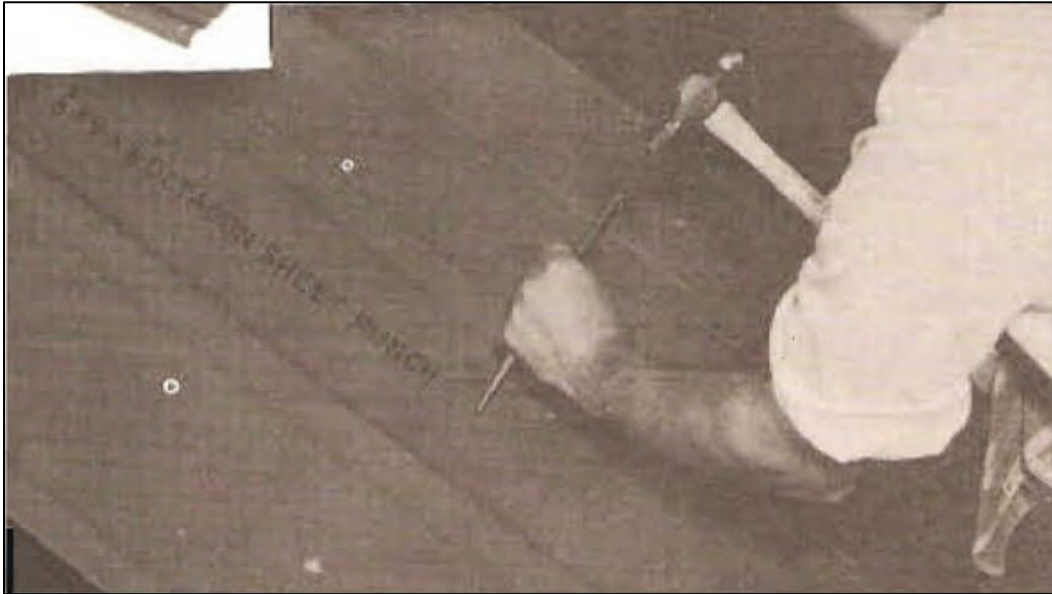
Figure 75. Depicted is the method used for field punching holes for a Butler prefabricated warehouse. Field punching would become unnecessary with the advent of self-tapping screws in the 1960s. (Butler Manufacturing Company, "U.S. Navy rigid frame utility warehouse building erection instructions for the 40'-0" x 100'-0" building," Kansas City, MO: Butler Manufacturing Company, 1945).
