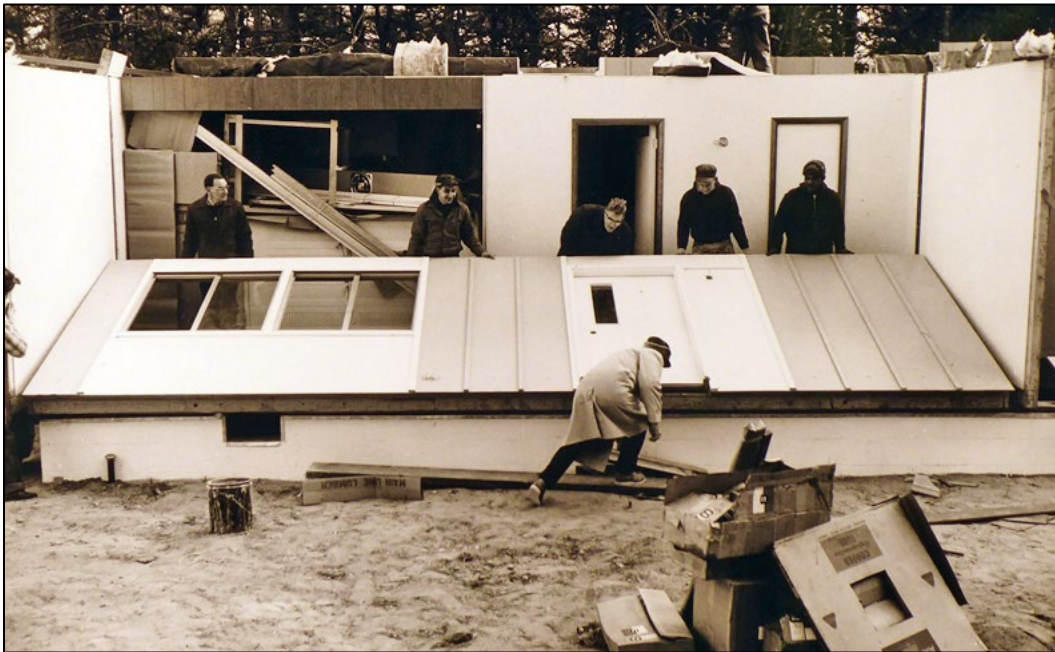
Figure 156. The ground floor front exterior wall is being lifted into place out of the shipping structure, Andrews AFB, Maryland, 1964 (NARA College Park, RG342-B).
