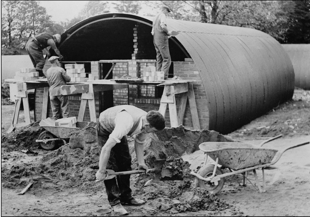
Figure 16. British civilian contractors erecting a Nissen hut, 1940–1946 (Library of Congress LC-USE6- D-008298 (P & P) LOT 3476).
