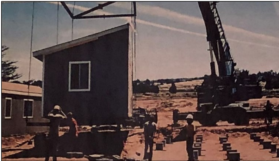
Figure 177. A modular section of housing being lifted into place by crane, Fort Ord, California, 1986 (E.R. Heilberg, III, “The Corps of Engineers: Leaders in Customer Care,” The Military Engineer 78, no. 505 (Jan.–Feb. 1986): 6–9).
