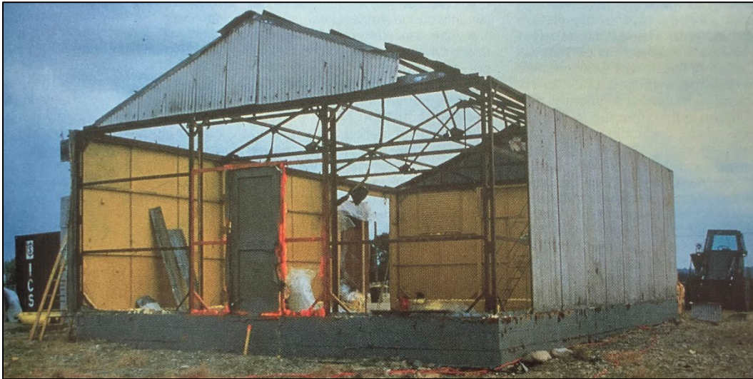
Figure 188. A metal prefabricated building in which a barrel of radioactive Americium 241 was discovered in 1986. The structure appears to be a Mesker Building due to the truss design combined with the pre-framed doorway and sidewalls, Wright Patterson AFB, Ohio, 1991 (Richard A. Phelps, “Environmental Management Offices: Key to the Air Force’s Future Viability,” The Military Engineer 83, no. 543 (July 1991): 44–46, 45).
