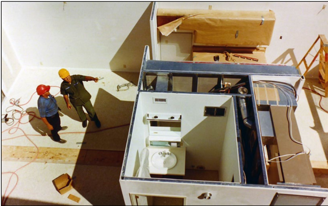
Figure 161. The utility core of one side of a modular duplex, George AFB, California 1971 (NARA College Park, RG342-B).
