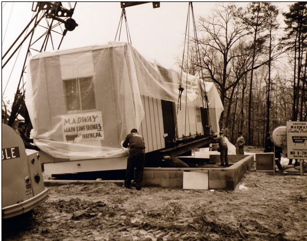
Figure 155. A Madway Main Line Homes house is being lifted into position on top of the foundation, Andrews AFB, Maryland, 1964 (NARA College Park, RG342-B).
