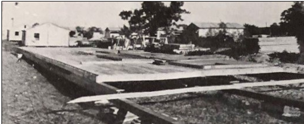
Figure 39. Floor panels of Bush Type-B building are being placed on the foundation, consisting of long horizontal wooden beams supported by wood footing (April 1943 advertisement for Bush Prefabricated Structures, Inc. (Clinton G. Bush Co., "The Bush Type 'B' All Purpose Building," Prefabricated Homes 1-5 (April 1943): 1).
