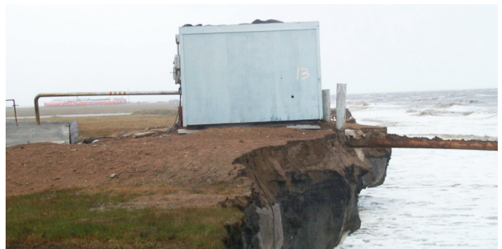
Coastal Erosion near an Air Force Early Warning Site. Source: US Air Force
