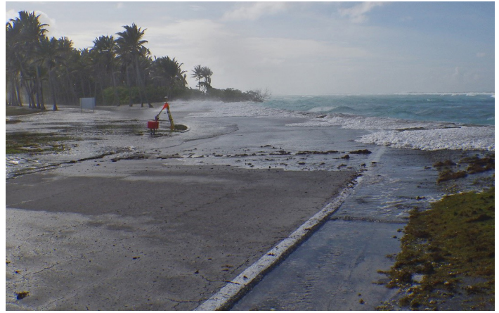
Waves wash over a road on Roi-Namur Island, Kwajalein Atoll, Republic of the Marshall Islands. Source: Peter Swarzenski
