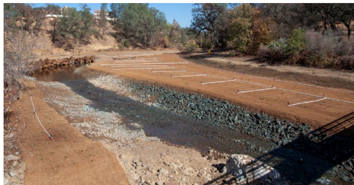
Post-construction at the former Beale Lake Dam site after removal, but before seasonal rains started at Beale AFB in October 2020. The area pictured used to be Beale Lake behind the dam, and is now a rocky, seasonal stream. Photo by Brandon Honig, USFWS, Sacramento, External Affairs Office.
