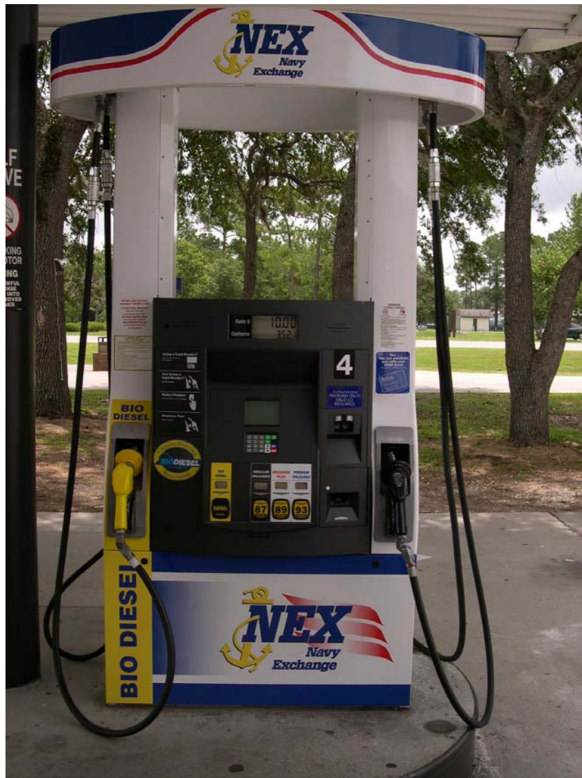
Figure 2. Biodiesel station at Navy Exchange at Kings Bay, GA
