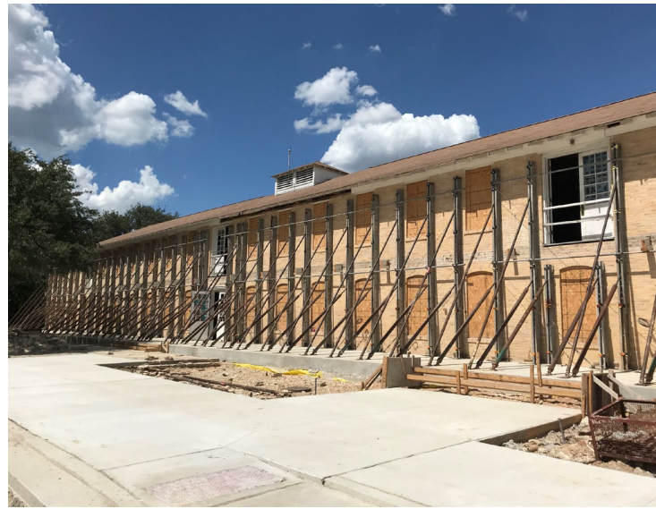
In process in the rehabilitation of historic Building 1. The building required significant structural support which required close coordination with the State Historic Preservation Office (SHPO) to proceed with stabilization plan.
