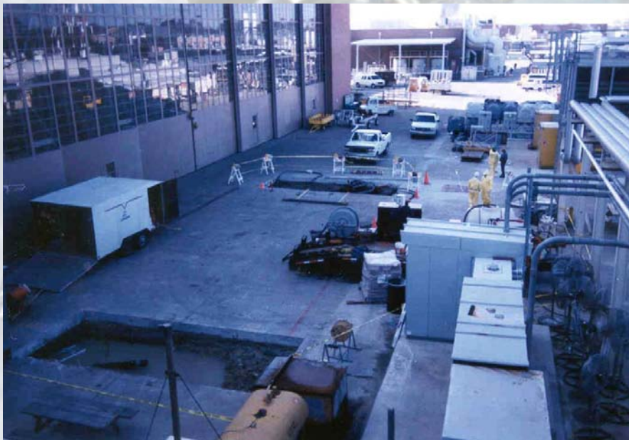
Restoration activities in Cherry Point's highly congested industrial area require careful coordination to limit impacts on production and avoid damage to utilities and infrastructure.
