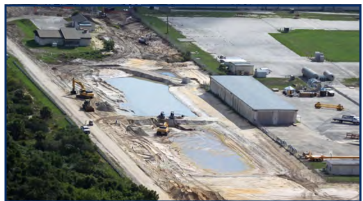
Larger hydrologic treatment basin during construction—Jun 09. An innovative sustainable approach to plume control!
