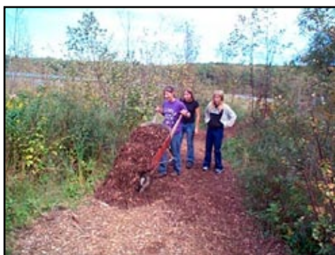
Little Falls High School students build a nature trail on Camp Ripley as part of a bog-walk project on National Public Lands Day.
