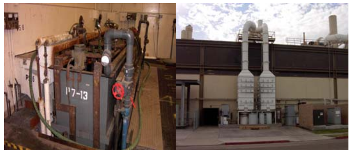
Figure 2 – Existing Chrome Plating Tank Push Pull Air Ventilation (l) and Air Pollution Controls (r)
