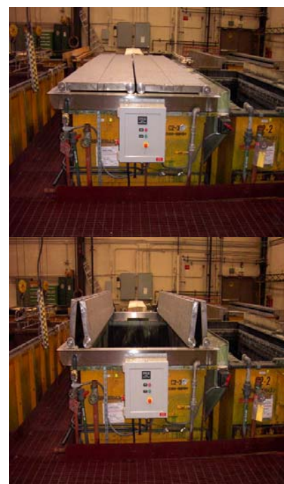
Figure 6 – New Automated Cover in the closed and open
