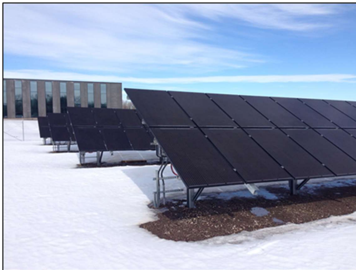
Sustainability Features of the newly constructed Arden Hills Division HQ include a 60 KW solar PV system, expected to meet 2.5% of the expected electrical load, daylighting, solar tube style skylighting, and a ground source heat pump system that will provide for all the heating and cooling needs of the building.
