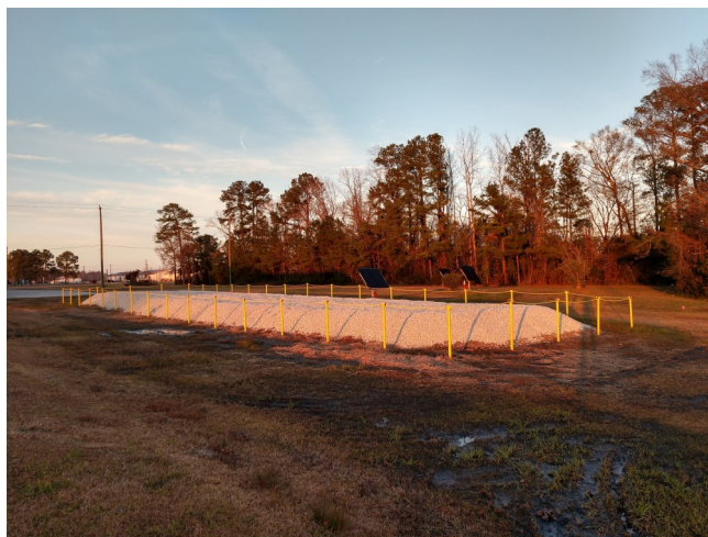
This subgrade biogeochemical reactor treated approximately 93,000 gallons of groundwater at Installation Restoration Program Site 93.
