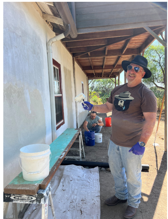
Successful collaboration with the DoW Cooperative Ecosystem Studies Unit Network has established a cost-effective pathway to restoration for the Las Flores Adobe NHL. The CRMP team worked with conservation specialists through University of Vermont to patch lime plaster cracks and apply a new coat of lime wash to the building's exterior. Pictured is Steve Harvey, archaeologist.
