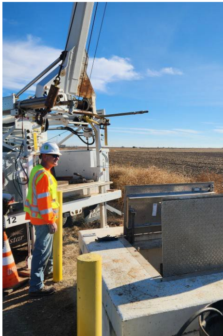
Extraction well redevelopment and rehabilitation have been key to maintaining the performance of the groundwater remedy.
